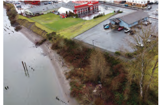
Before River Walk Installation w/ Massive Erosion
